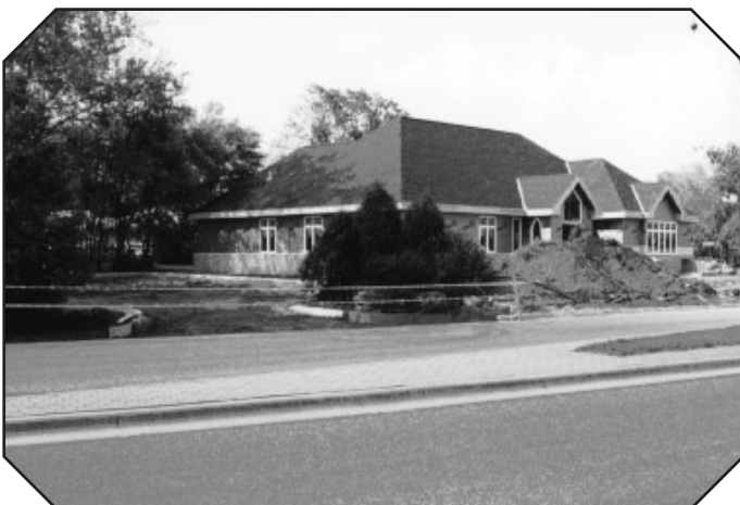
Parking lot on the west side of building, prepared for laying of blacktop
